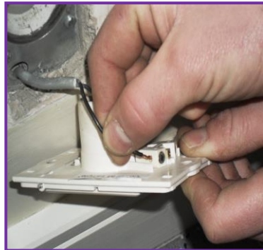
5. Remove trim plate from inlet and reattach LV cabled from old inlet.
